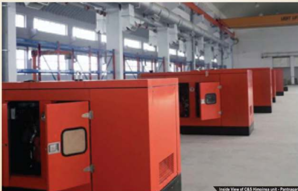
Inside View of C&S Himoinisa unit - Pantnagar
